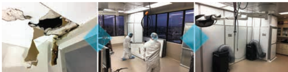
From top: Assessment and remediation of water damage being performed in a temporary STARC containment system. > Remediation and renovation performed with a STARC containment system and negative air.
