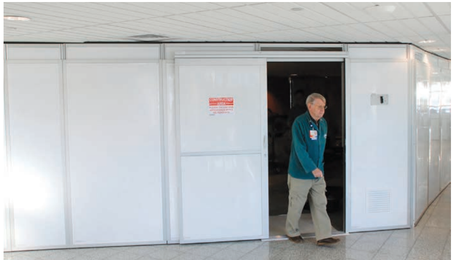
To comply with the ICRA requirement, the renovation required building a 100-foot airtight containment barrier around the construction zone.
